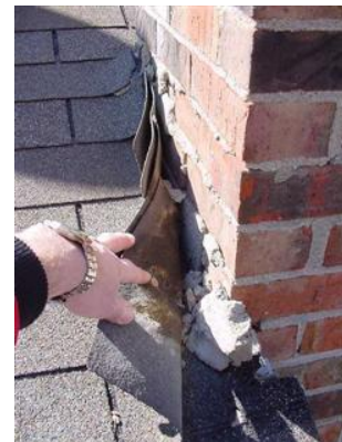
At right: The flashing is missing. The shingles continue up the sides of the chimney and were foamed in place.
