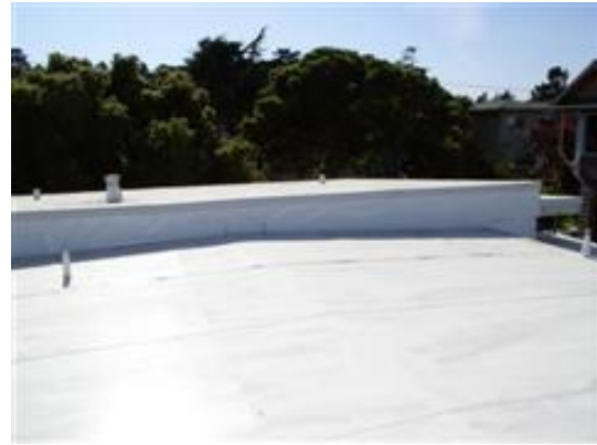
Above: This is another EPDM membrane. Notice the wrinkles between the sheets. This could easily allow water penetration. These areas need full evaluation.
