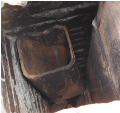
At left: This flue has collapsed due to a chimney fire. The installation of two flues not separated by a brick divide would no longer meet code for new construction.
