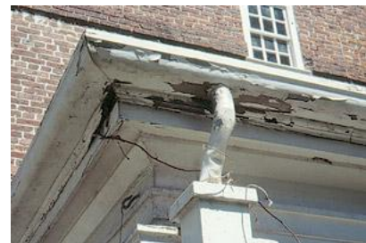
Above: a section of cornice guttering with visible rot; notice the downspout hidden within the column
