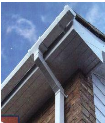
Above: standard vinyl guttering, properly installed
