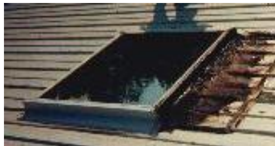
Below: A skylight in a metal roof shows damage to the roof on the top-side.
