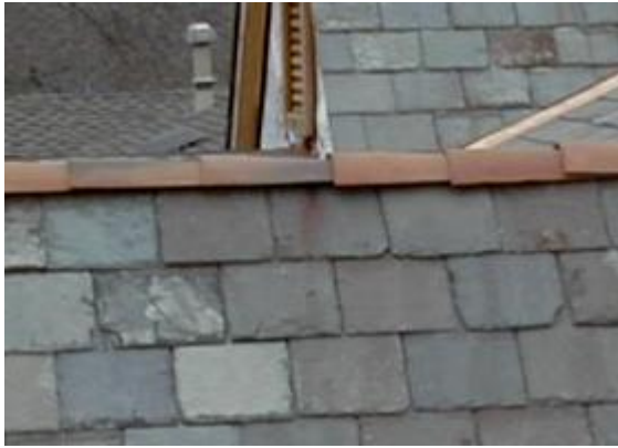
At left: an older roof; small chips at the corners of tiles are generally not of concern. Note the ridge cap, which is made of clay tile.
