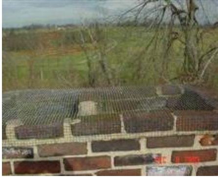
Above: This chimney has no cap or liner all. It is no longer legal to build an unlined chimney.
