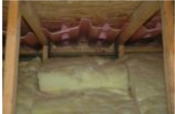
Above: Poorly installed insulation is blocking the soffit vents. Also, the baffles are incorrectly installed. (Courtesy of John Hastings)
