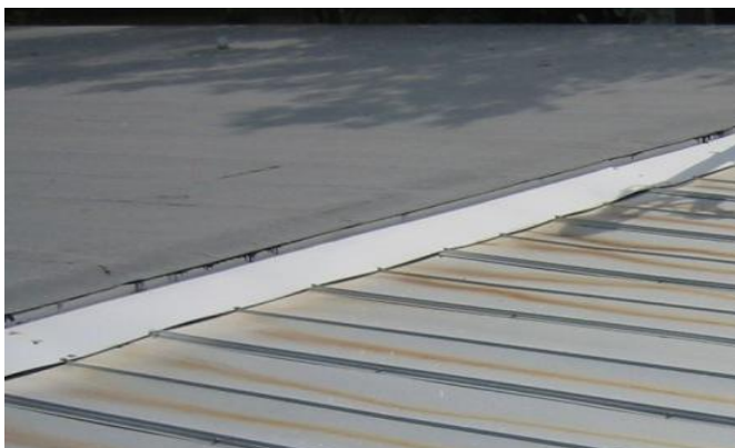
The photo at left shows both poor flashing between surfaces and improper use of 3-tab shingles on the lower roof.
