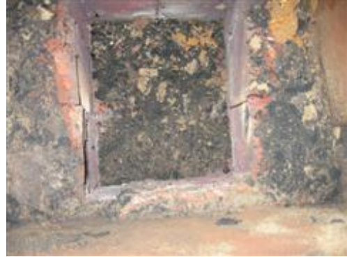
Above: This chimney flue has poorly done brick work and is filled with debris. (Courtesy of Joe Myers)
