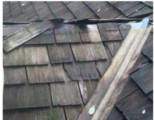
Above: shingle ridge detail showing broken shingles and considerable erosion; also note the open W-valley flashing. (Courtesy of Pat Dacey)
