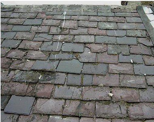
At left: an older slate installation showing many broken and dislodged tiles
