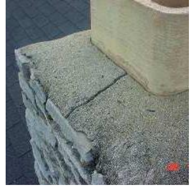
Above: cracking in the chimney cap
