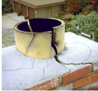
Above: Cracking can be seen both in the liner and in the chimney cap. This damage was caused by a flue fire.
