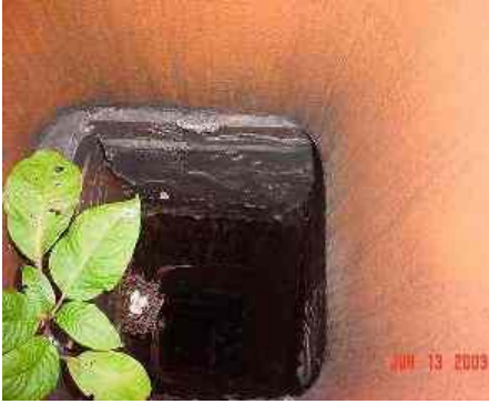
Above: This is the view down an unlined chimney flue. Vegetation is growing through it, and a bird has built its nest in it, too.
