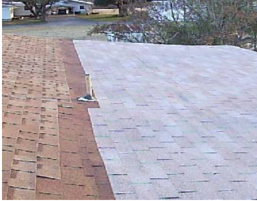
Above: another example of poor flashing between surfaces and improper use of 3-tab shingles on the lower roof
