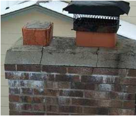
Above: The flue on the left has been sealed with concrete, and the flue on the right has a rain cap. However, the chimney cap itself is cracked and the brick work is showing signs of efflorescence.
