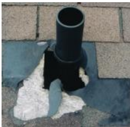
Above: This is a plastic vent flashing which was damaged by raccoons.
