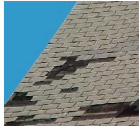
Above: a fiberglass asphalt shingle roof whose shingles became brittle over time, allowing the wind to get under them and blow them off the roof
