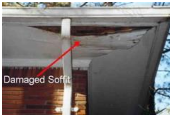
Above: This kind of damage is a typical sign of previous ice damming in some climates. (Courtesy of Mike Rose)
