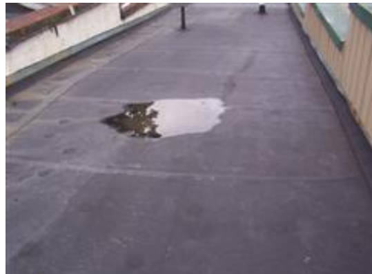
At right: This is an EPDM membrane covering. The ponding should be reported.
