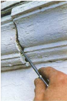
At left: Wood rot has loosened the cornice molding and is splitting around the nails.
