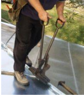
At left, At an installer is crimping together the seams on a metal roof.
