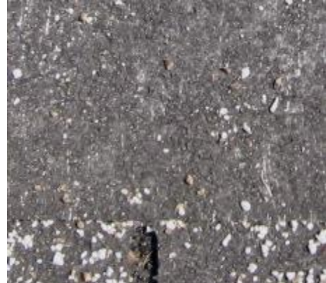
Above: an extreme close-up of a badly weathered fiberglass-based shingle whose fibers are exposed
