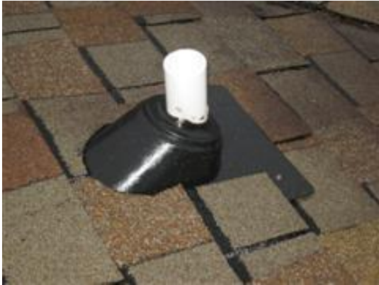
At left: This plastic vent flashing has been installed upside down. This will probably allow moisture to travel down the outside of the vent pipe.
