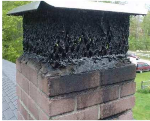
Above: This rain cap is completely choked with creosote, which is not unusual to find when the homeowner has been burning unseasoned timber.
