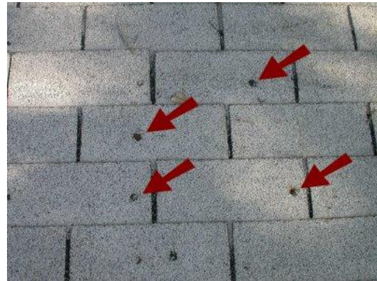
Above: Nail pops indicate where the fasteners have backed out of the roof.
