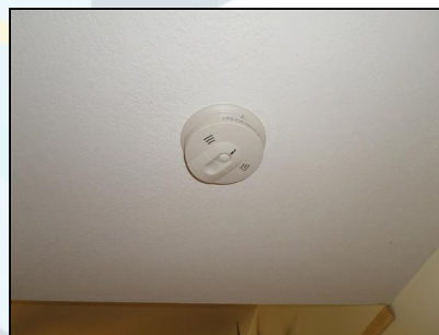
6.16 Item 1(Picture) Smoke detector
