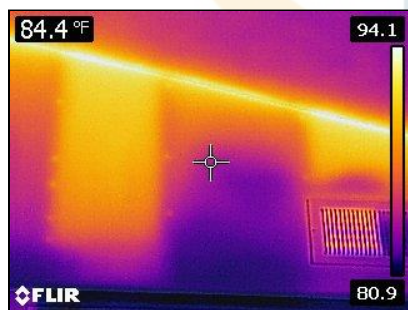
2.5 Item 2(Picture) Yellow area is missing insulation
