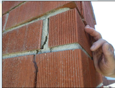
1.6 Item 2(Picture) Cracks
