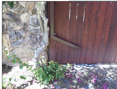
1.4 Item 2(Picture) Downspout too high
