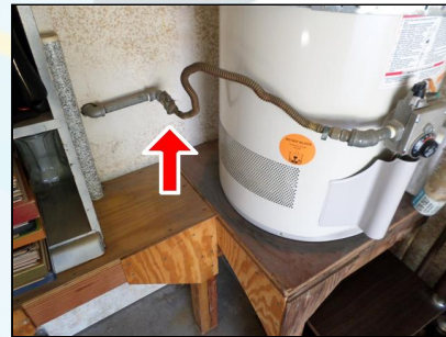
7.4 Item 2(Picture) Shut-off
