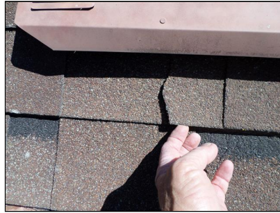
1.2 Item 2(Picture) Torn roof material
