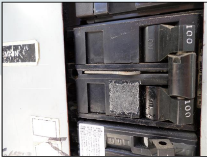
6.6 Item 1(Picture) Main breaker
