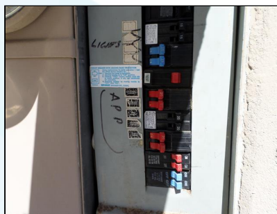
6.7 Item 2(Picture) Breakers
