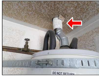
7.4 Item 4(Picture) Possible asbestos
