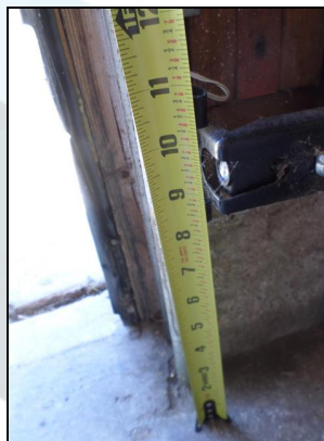
9.0 Item 1(Picture) Sensor too high
