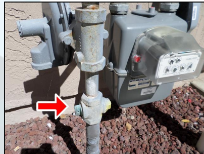
7.5 Item 1(Picture) Gas shut-off
