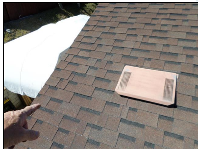
2.3 Item 1(Picture) Roof vent
