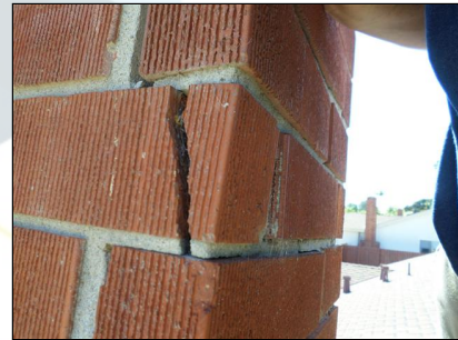
1.6 Item 3(Picture) Cracks
