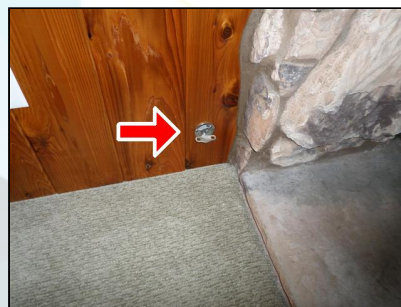
8.0 Item 1(Picture) Shut-off
