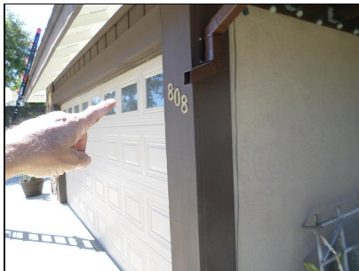
1.4 Item 1(Picture) Downspout too high
