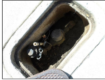
7.2 Item 1(Picture) Meter & shut-off
