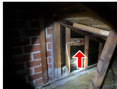
2.4 Item 1(Picture) Improper Wire Termination
