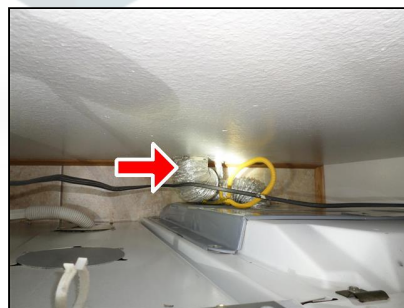
7.5 Item 2(Picture) Shut-off for dryer
