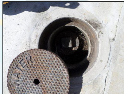
7.3 Item 1(Picture) Sewer clean-out
