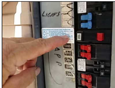
6.7 Item 1(Picture) GFCI breaker
