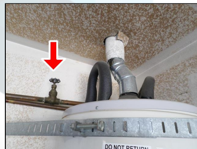
7.4 Item 3(Picture) Shut-off
