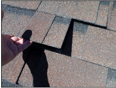
1.2 Item 1(Picture) Not sealed
