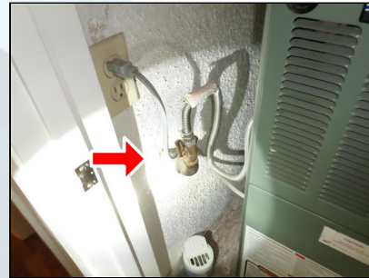
5.2 Item 1(Picture) Shut-off
