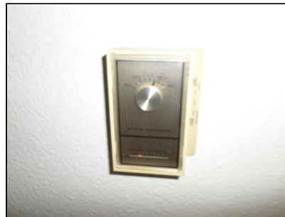
5.3 Item 1(Picture) Thermostat
