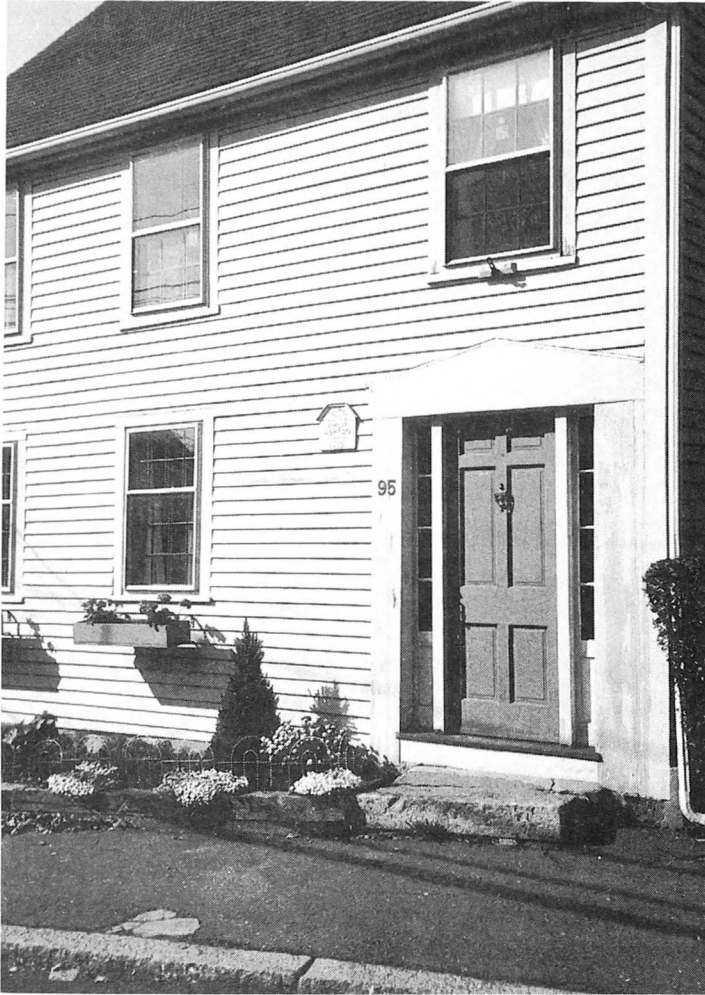
Fig. 5-1. A well-built and properly maintained building will last longer than anyone can estimate, as attested to by this building built in 1715.
