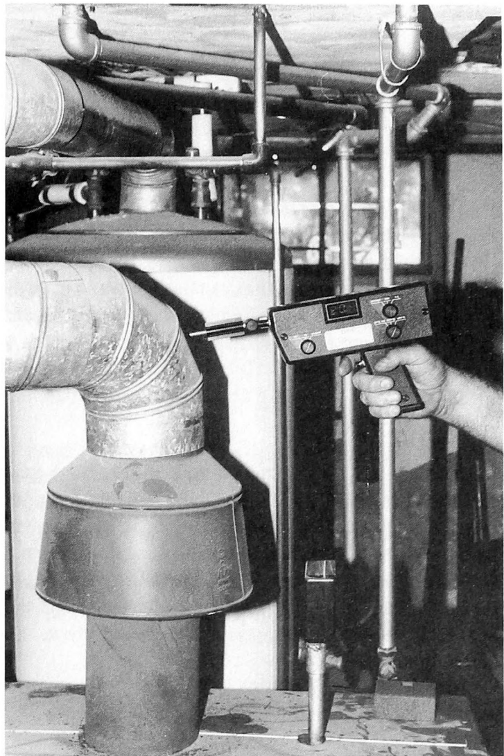
Fig. 7-14. Once a year have your serviceman perform an energy efficiency test on your system. Testing equipment can save you money in the long run.
