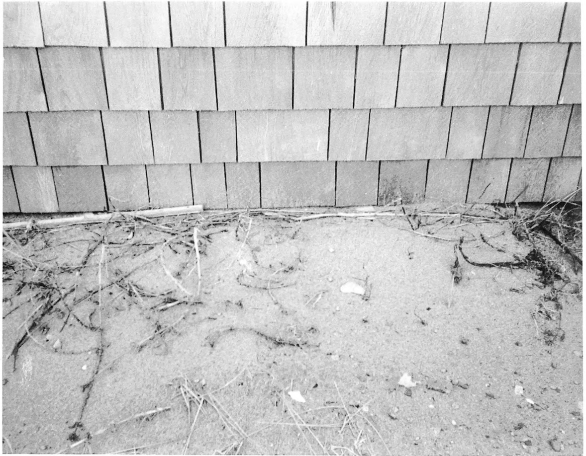
Fig. 5-4. Wood in direct contact with soil will rot out in time unless it is pressure-treated wood. The photograph shows how moisture can be drawn to the wood and how easy it would be for wood-boring insects to start their trek.
