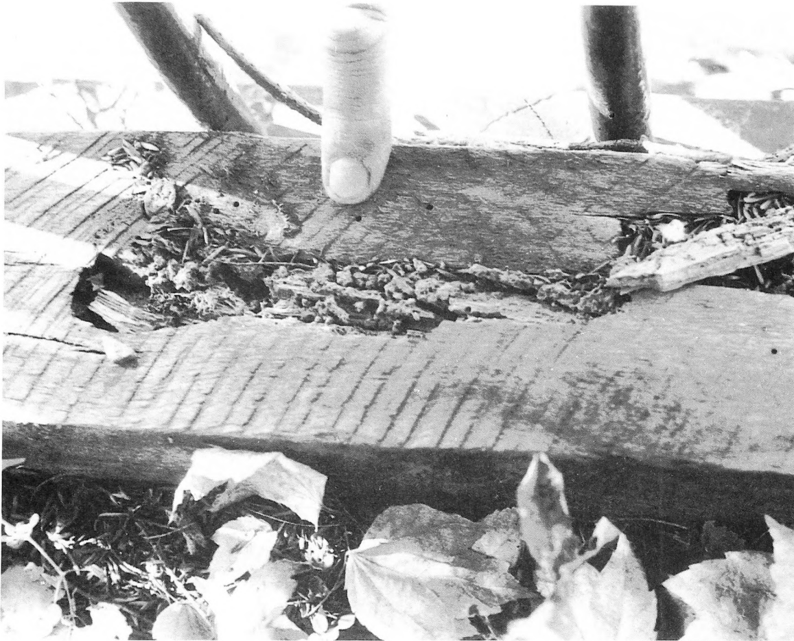
Fig. 5-17. Wood damaged by powder-post beetles.
