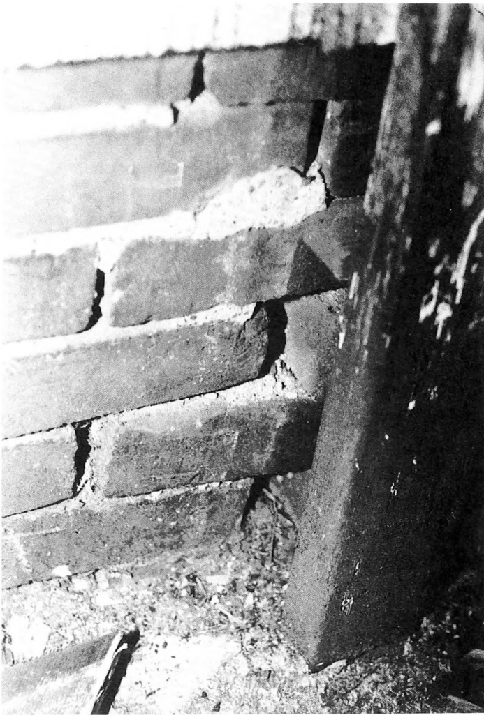
Fig. 1-19. Major damage to mortar joints and displacement in masonry materials will cause structural damage and water penetrations to the buildings.
