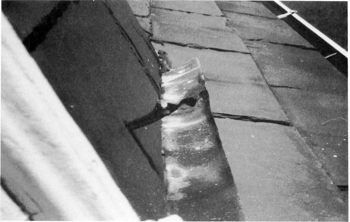
Fig. 1-2. Old and damaged flashing is probably one of the major entry points for water. If you find such deteriorated areas, be sure to either repair or replace them.
