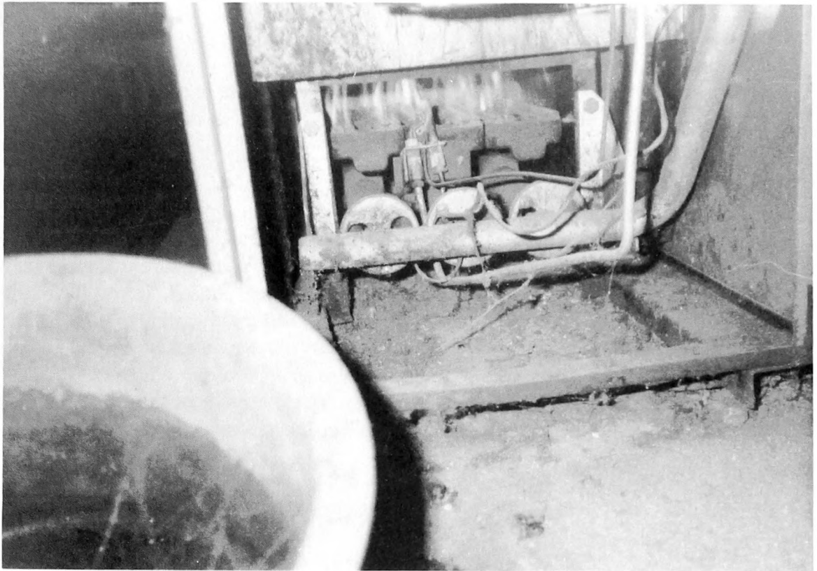
Fig. 3-21. Dirty heating systems that need service means that the owner is not keeping up with maintenance chores. For a nominal fee you can have your heating system tuned up on an annual basis.
