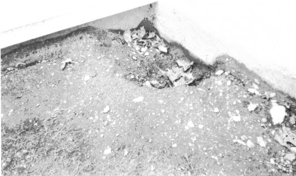
Fig. 2-4. Depressions and low spots along foundation walls will result in seepage into the basement areas. Regrade all low spots so that water will flow away and not towards your building.
