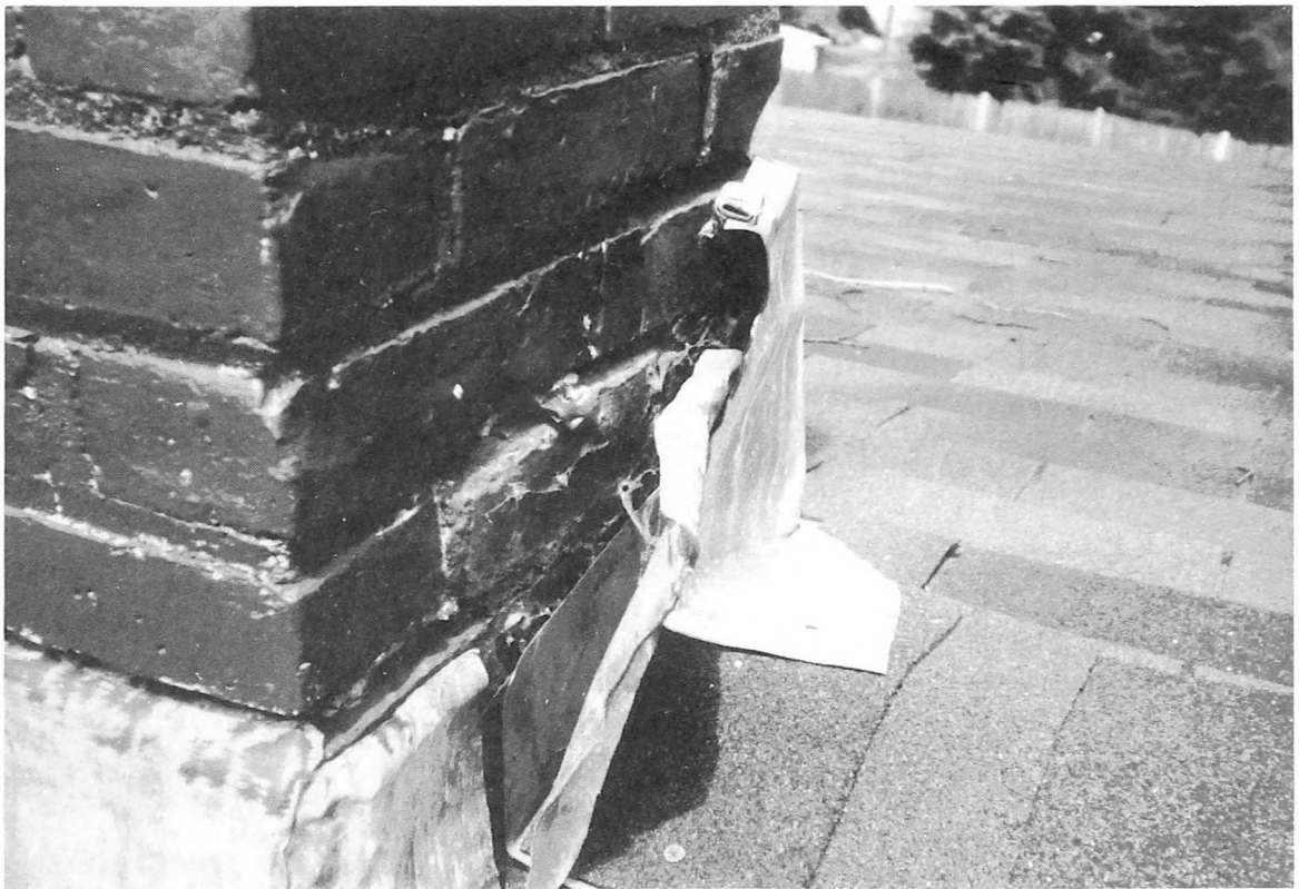
Fig. 4-11. Inspect and maintain flashing areas to avoid open areas such as this, which will result in major leaks to the building.
