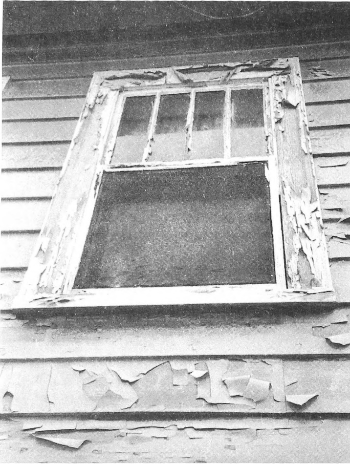
Fig. 6-1. Tight houses with minimal or no ventilation will often have excessive peeling paint and decaying wood from too high a moisture content in the wood.
