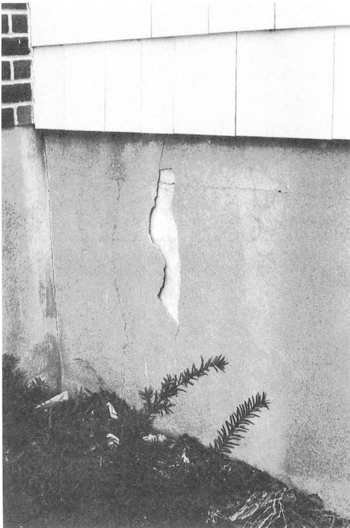
Fig. 2-16. Be sure to tap out loose sections of stucco so that the areas all are flush to each other. Recement and seal up any such damaged areas before they increase in size.
