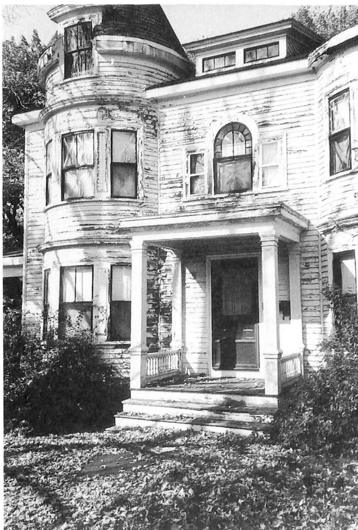
Fig. 5-2. A poorly maintained building will deteriorate long before it should. Remember, maintenance is the key to a healthy building.
