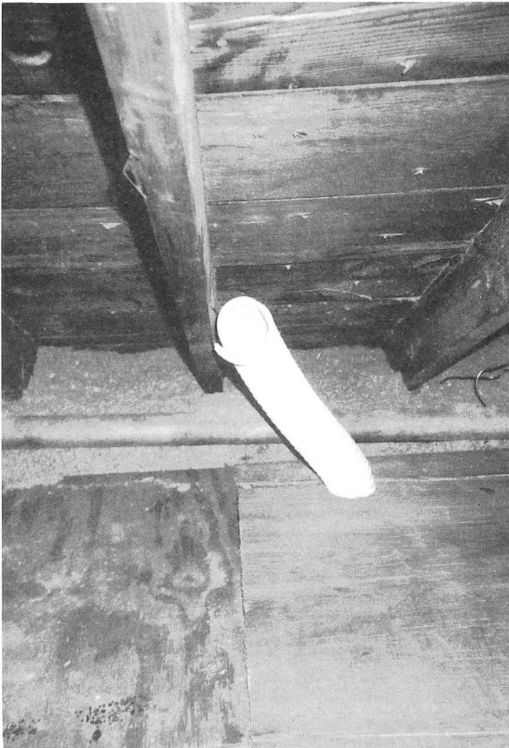
Fig. 3-14. Never vent dryer vents into enclosed spaces such as attics or crawl spaces. The resulting moisture buildup will cause decay and damage to both framing and insulation.
