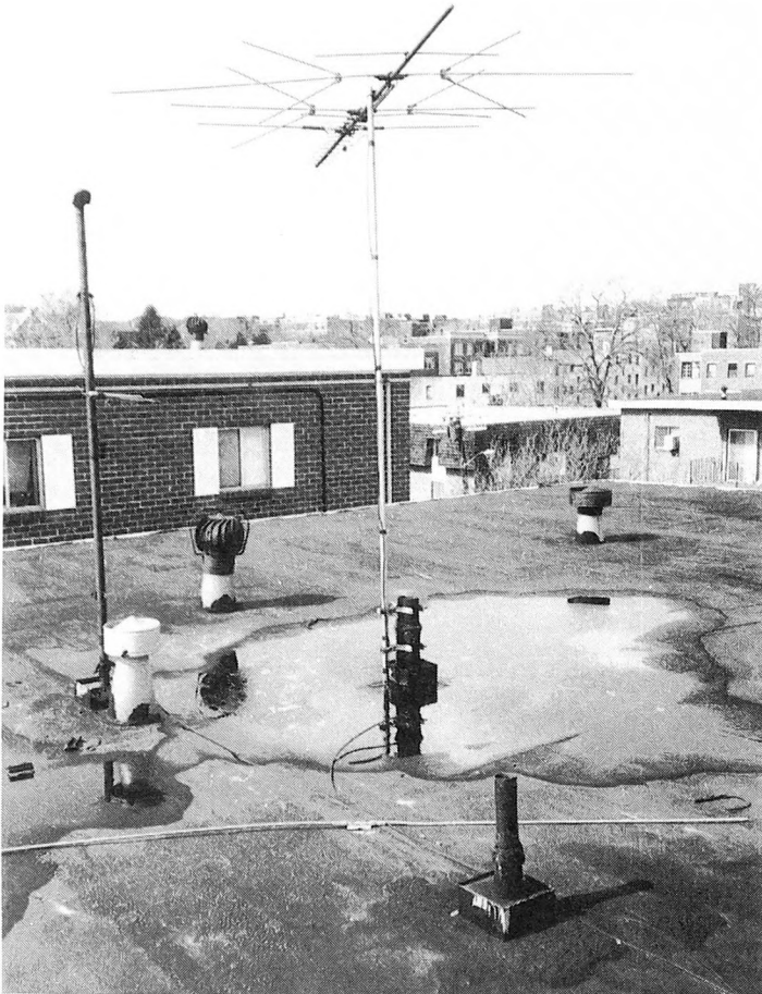
Fig. 4-15. Avoid attaching antennas to chimneys and vent pipes. Damage to flashing areas and eventual leaks will result.
