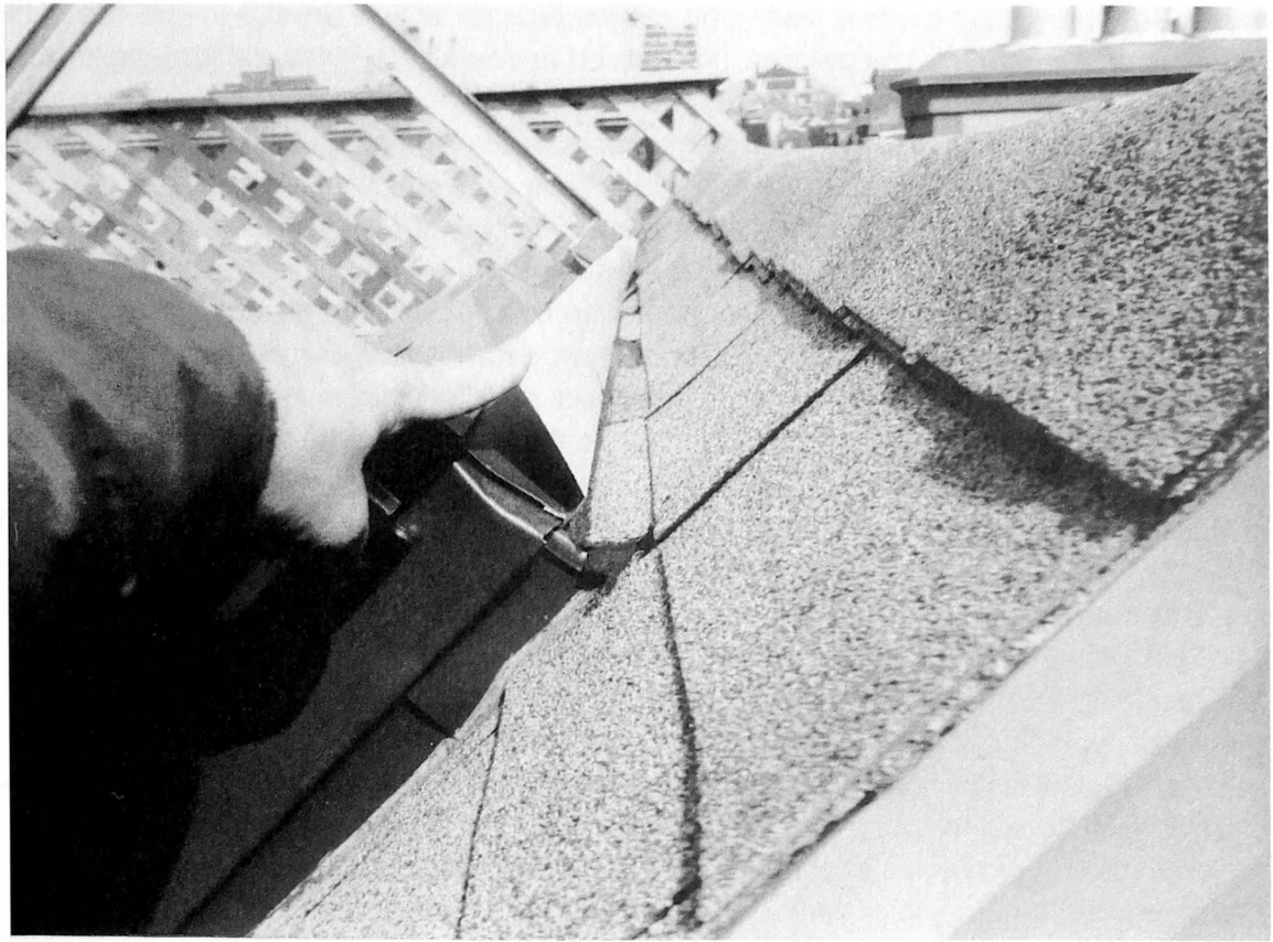
Fig. 4-16. The flashing is not under the shingles as it should be. The results could be leaks to the building.
