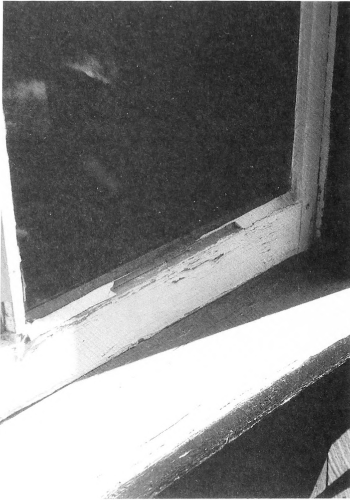
Fig. 1-6. Failure to maintain windows will result in damage to the windows and deterioration to adjacent building components.
