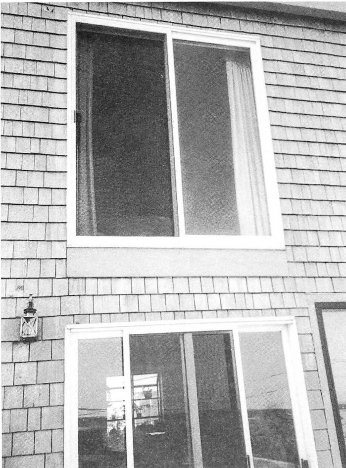
Fig. 8-29. Any sliding door, opening, etc., that opens out must have a platform or safe stairways. Make sure that any unfinished projects are safely secured to prevent an unwarranted accident.
