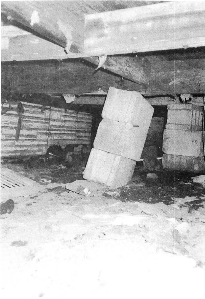
Fig. 1-15. Inspect crawl spaces once a year and make corrective repairs and maintenance work to avoid structural damage.
