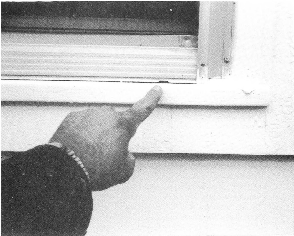
Fig. 6-2. Open up or provide weep holes in all storm windows to allow trapped moisture to escape before it can do any damage.
