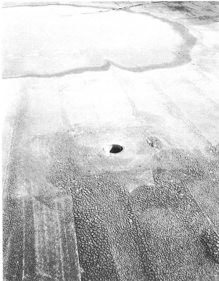
Fig. 4-17. Flat roofs without screen covers for drains will, in time, accumulate more than water in the drains.
