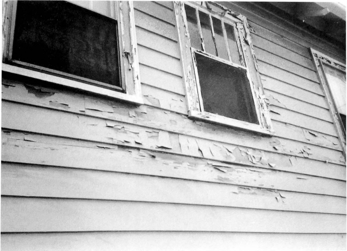
Fig. 3-18. Severe peeling of siding and trim areas as well as decay to wood are usually the results of buildings that are too tight and lack sufficient ventilation.
