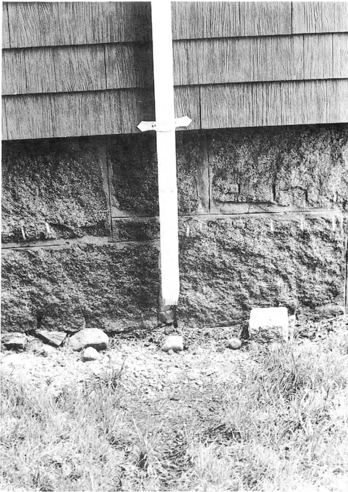
Fig. 1-4. Roof drainage that discharges directly to the foundation grade will eventually result in wet basements. Provide extensions to carry water away from the foundation walls.
