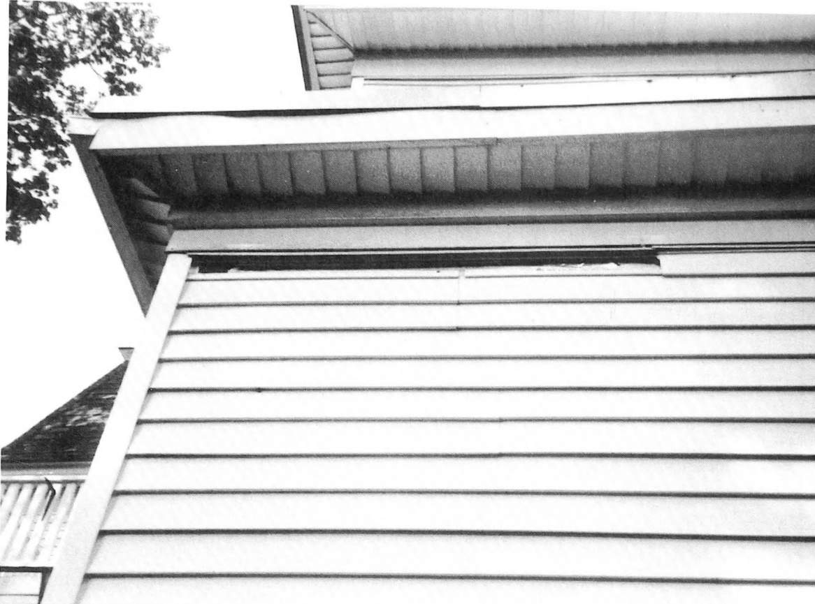
Fig. 4-29. Mysterious leaks into the building might not be the result of a defective roof. The entrance area could be the siding.
