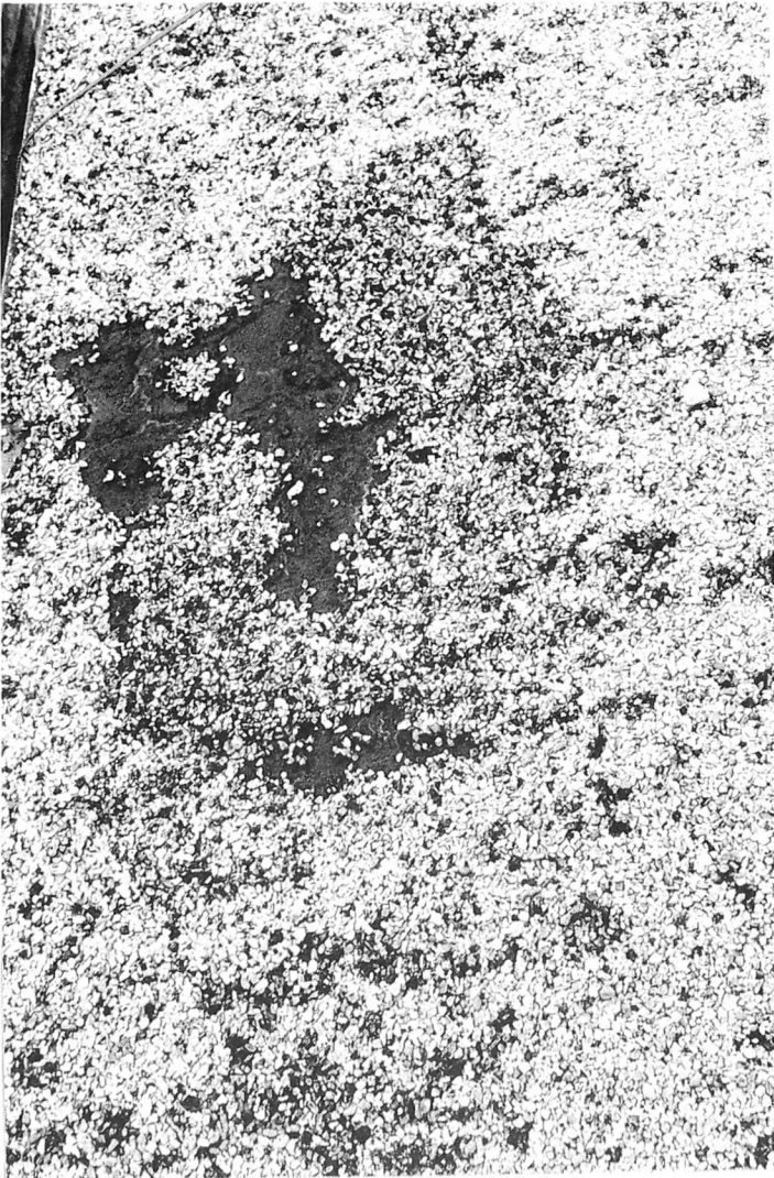
Fig. 4-6. Roofs are not meant to be walked on except in emergencies such as repair work. Damaged finished surfaces are usually the result of unwarranted walking on roof surfaces.
