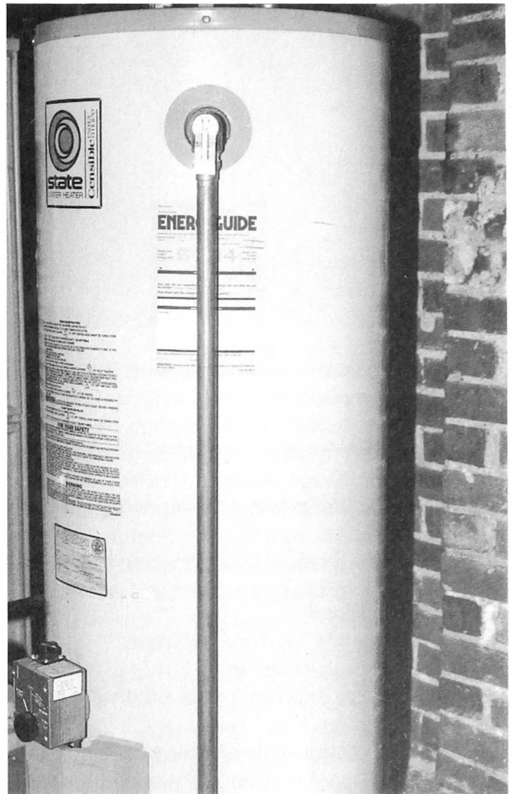
Fig. 7-30. The temperature relief valve on the right side of the tank. Note the drip pipe connected to it; it will discharge water to the floor and not at anyone standing next to the tank.
