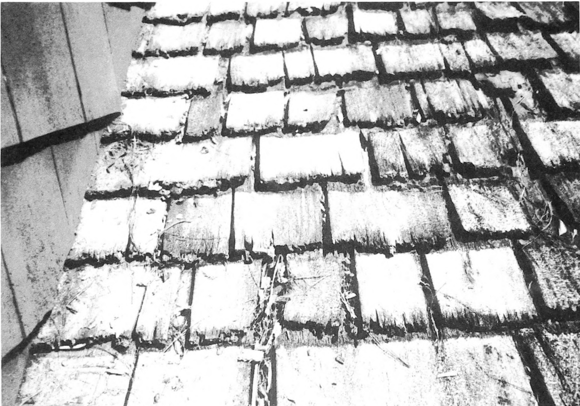
Fig. 4-27. Advanced stage of roof failure. This roof is well beyond its useful life expectancy. Leaks to the interior have probably been occurring for years.
