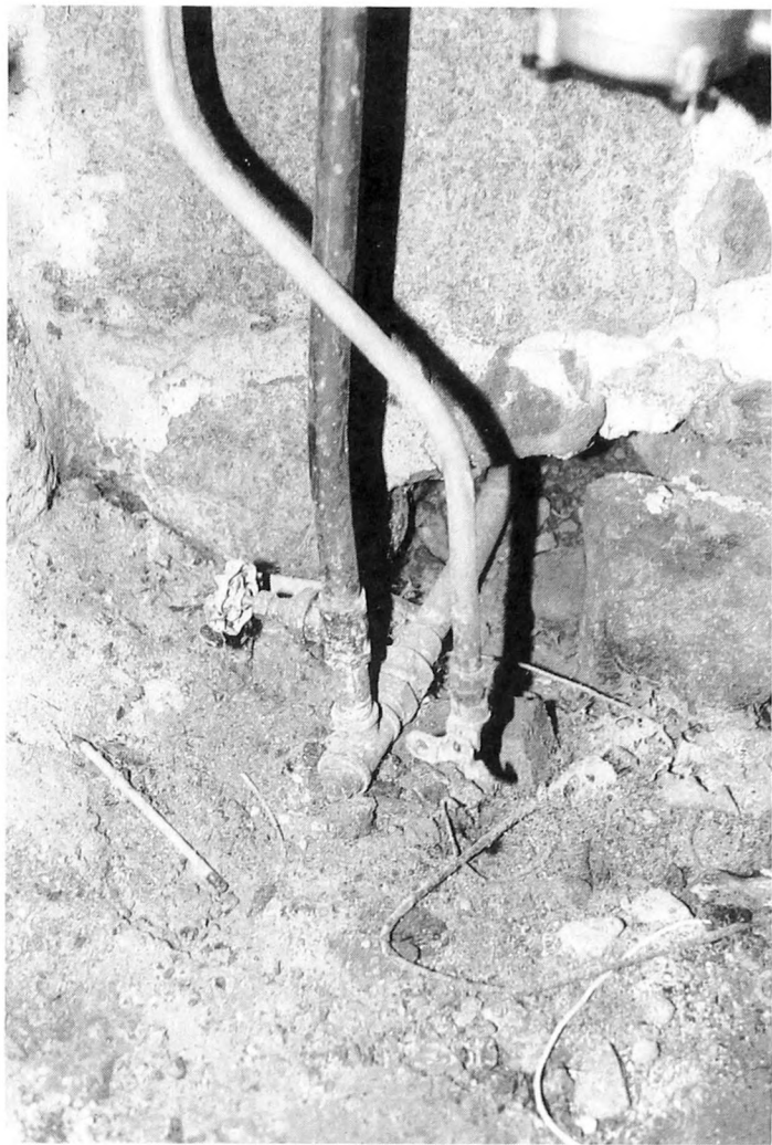
Fig. 1-20. During your inspection-maintenance tours, be sure that the grounding connection is secure to the main water pipe and not disconnected as seen in this photograph.
