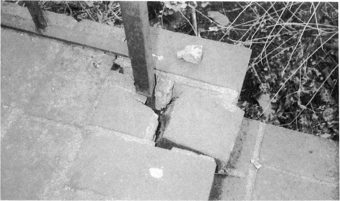
Fig. 8-26. Loose connections for posts or railings require immediate attention and repairs.
