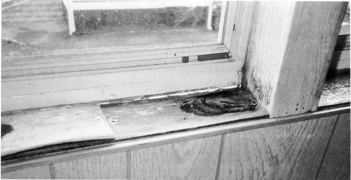
Fig. 3-24. Storm windows without weep holes could cause condensation, resulting in discoloration and decay in trim areas.
