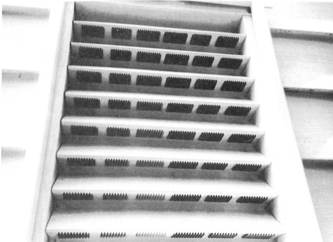
Fig. 3-3. By having minimal ventilation in a building, you create the same situations for condensation that no ventilation causes. New technology is not always an improvement as seen in this newer type gable vent. The surface areas for air movement are restricted by the design of this vent.
