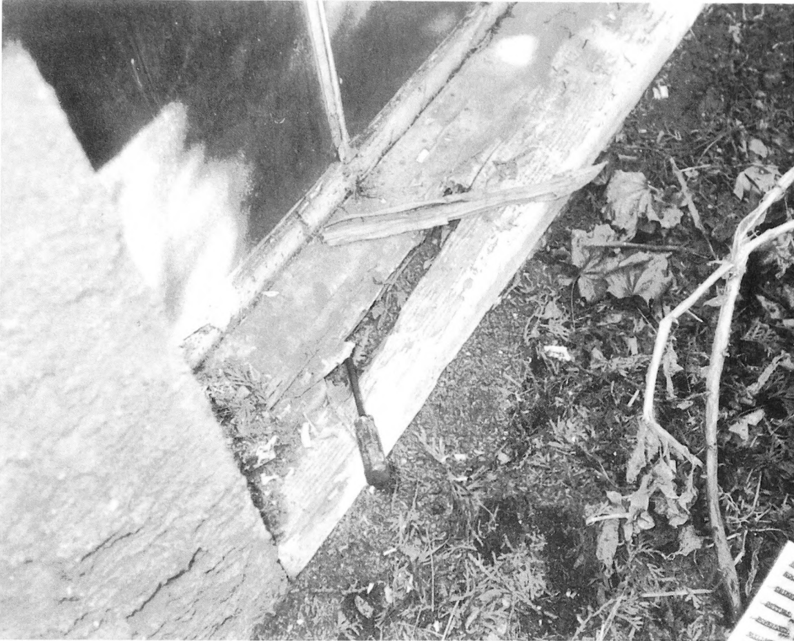
Fig. 5-19. Carpenter ant damage in a a foundation window sill.
