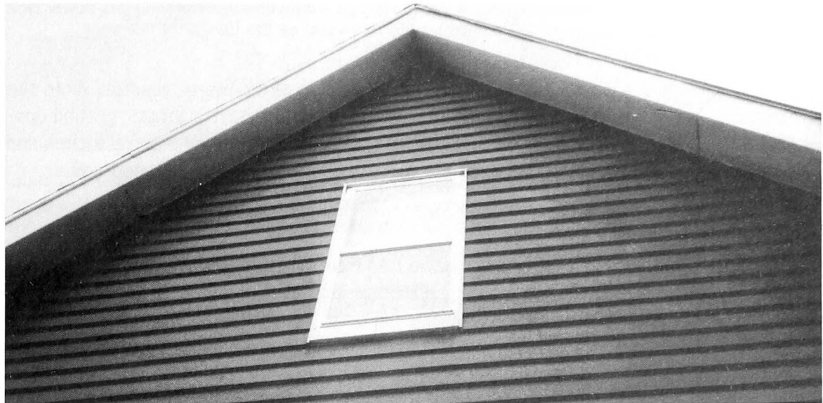
Fig. 3-2. Having no ventilation in a building is like wrapping your entire body in a plastic sandwich bag. The problem is compounded here by the vinyl siding. Concealed and visible condensation is rampant in this building.
