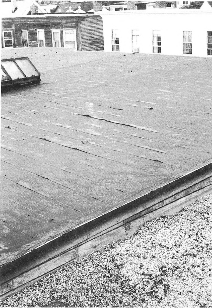
Fig. 4-2. Flat roofs tend to discharge water at a slower rate than pitched roofs, and hence some leakage into the building is likely—particularly if the roof is old and deteriorated.
