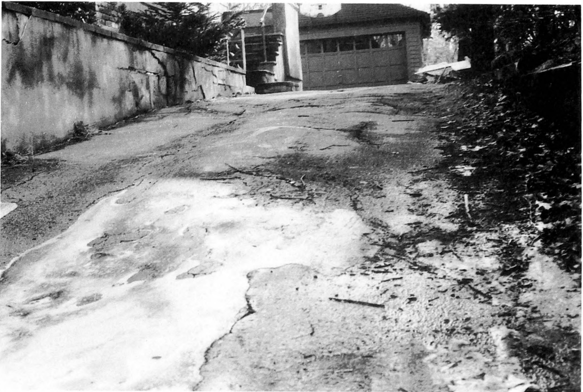
Fig. 1-13. Annual maintenance and repairs can help you avoid major costly driveway resurfacing.
