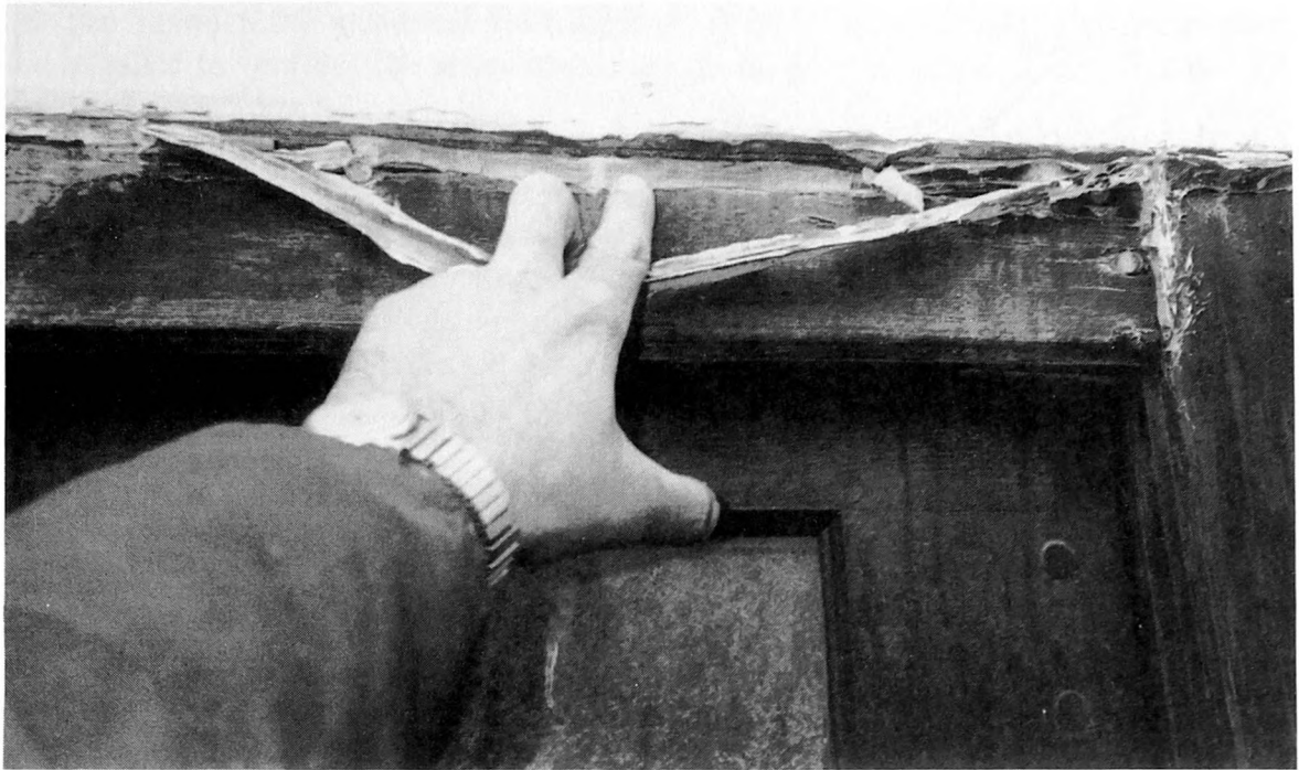
Fig. 6-4. Weatherstripping on doors, in this instance a garage door, should be monitored and repaired on an annual basis.
