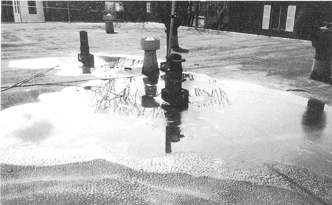
Fig. 4-3. Ponding of water on flat roofs not only results in leaks but also, in some instances, damages the roof structure.
