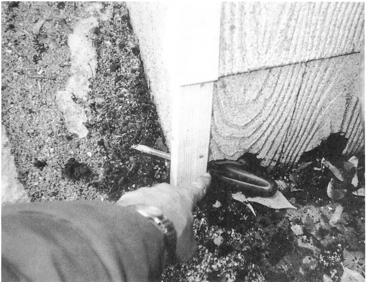
Fig. 5-10. Always be on the alert to any areas that have direct wood-soil contact. As you can see, the corner support post appears to have rotted out.
