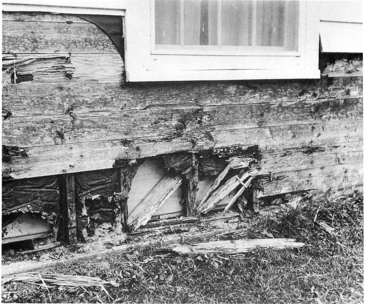
Fig. 5-18. Damage of the magnitude illustrated in this photograph requires the expert opinion of a structural engineer as to whether the building is still sound. (Courtesy of U.S. Forest Service)
