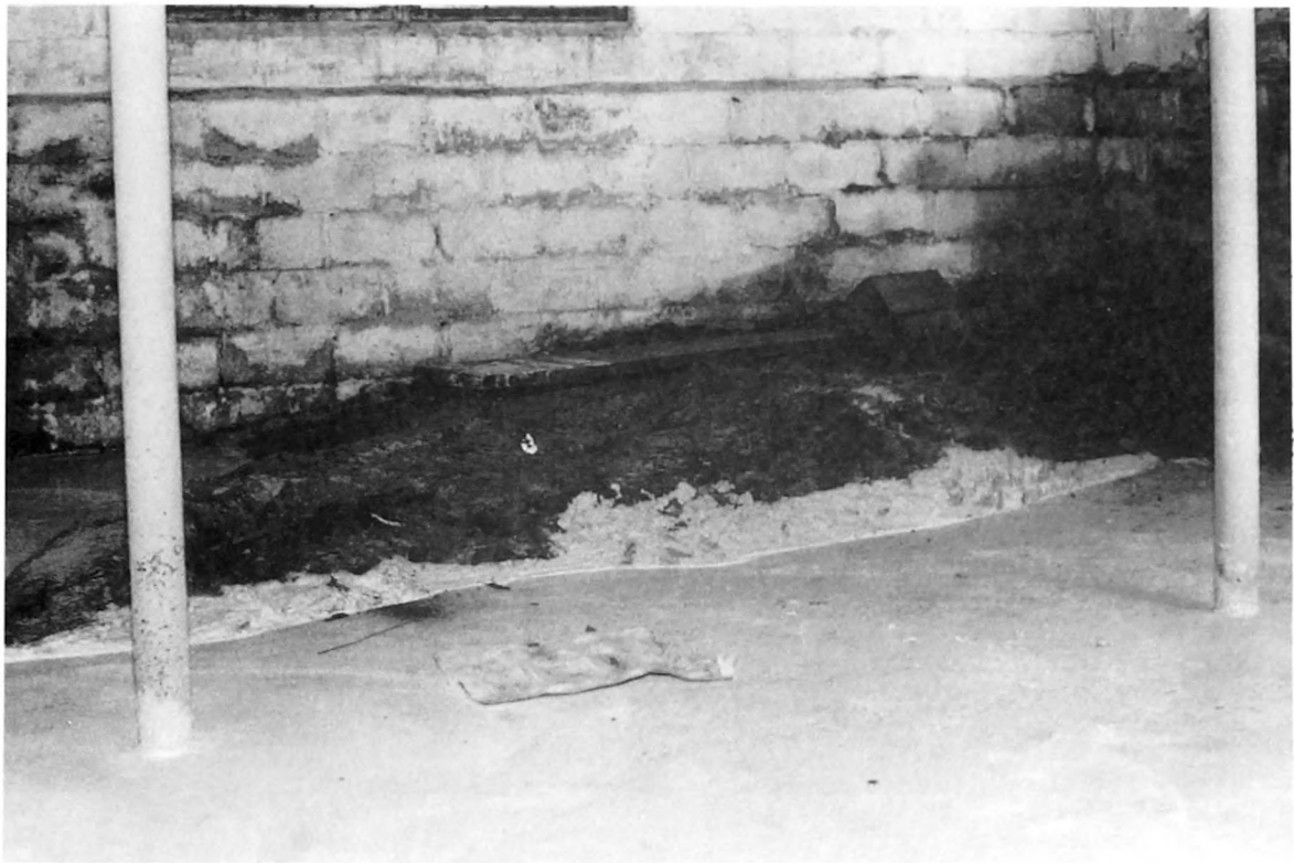
Fig. 2-8. Foundations that are built on and over ledge formations will usually be the recipient of unwanted water. By maintaining foundation grading and roof drainage runoff, you might be able to curb the amount of water seepage.
