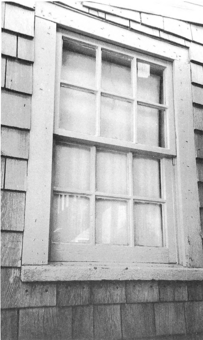
Fig. 3-23. Single pane windows will result in both heat loss and moisture transfer from the exterior. If you presently have such windows, consider having storm windows installed.
