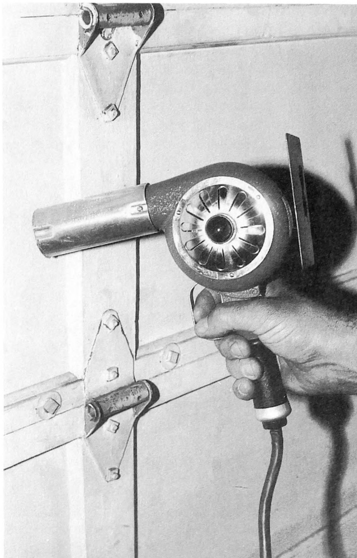
Fig. 8-2. Heat guns can help in removing lead paint in a relatively safe way. (Be sure to provide ample ventilation.)
