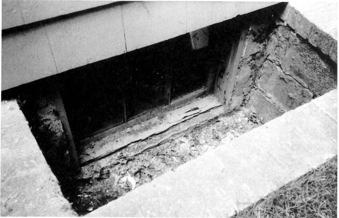
Fig. 2-5. Deep well foundation windows without protective hood covers will end up with what you see here—decay, wood-boring insect activity, and water in your basement.
