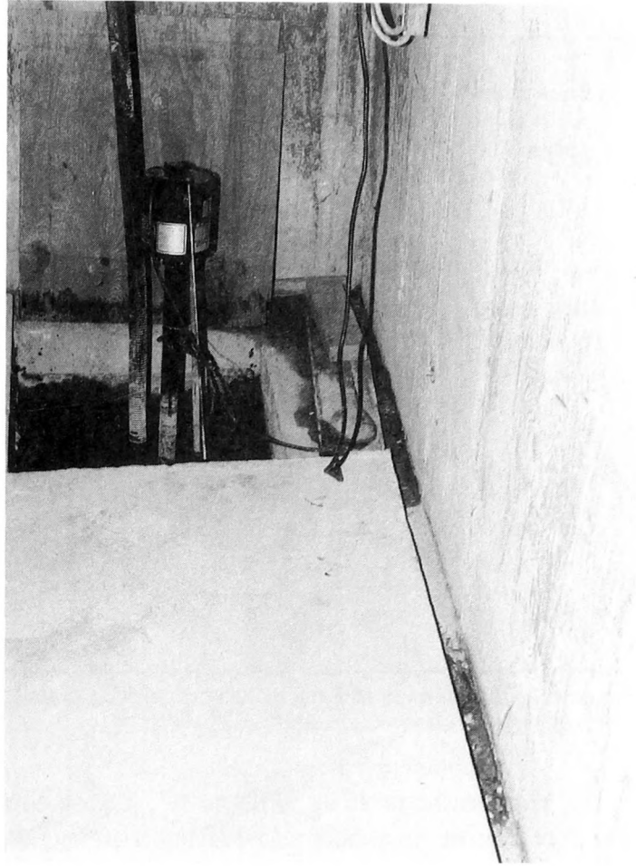
Fig. 2-21. This older form of interior perimeter drainage system is simply an open trench that leads water to a sump pump. The water is discharged out of the building, usually several feet away.
