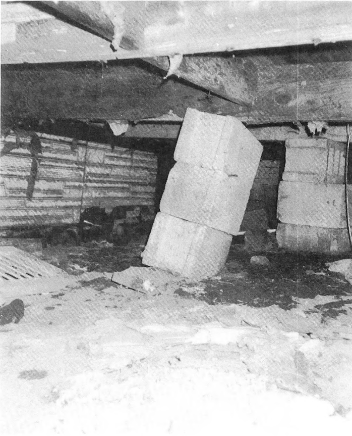
Fig. 3-9. Crawl spaces with exposed soil need vapor barriers on the soil to control moisture movement in the crawl space.
