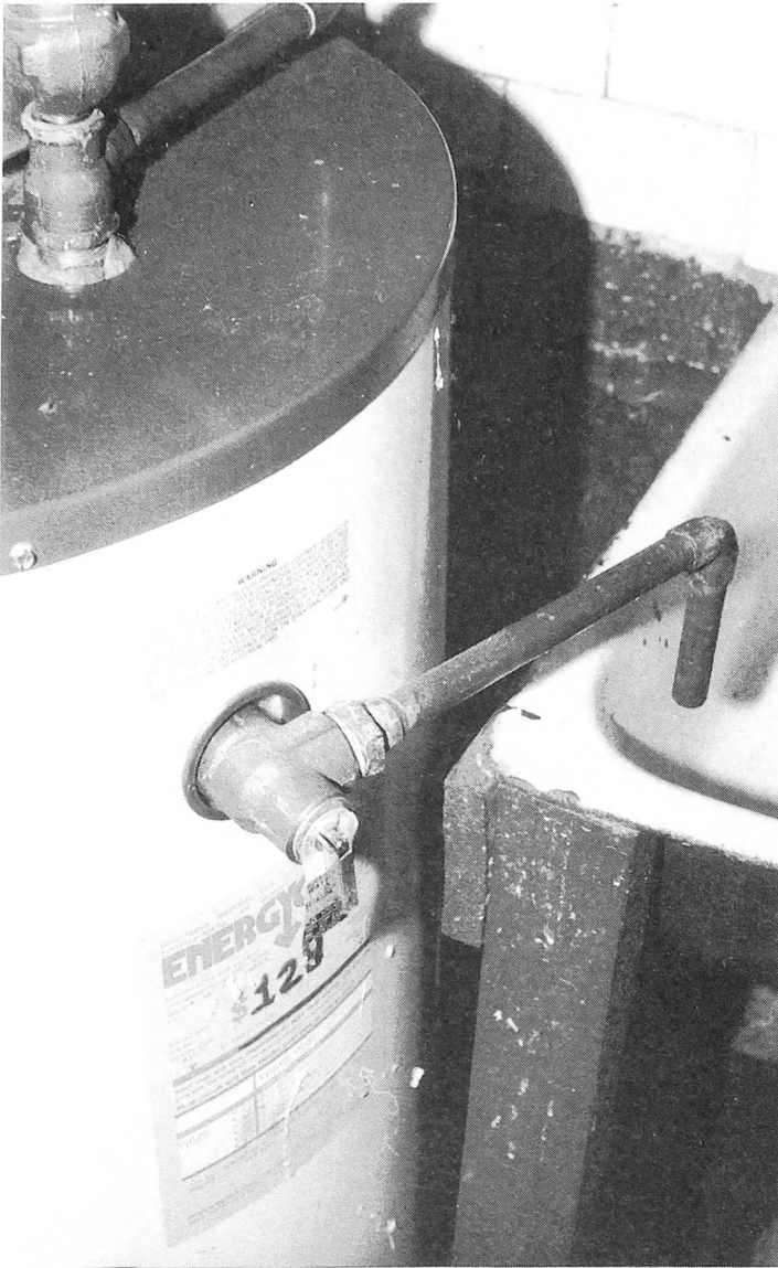
Fig. 7-31. Ideally the drip pipe of the relief valve should be discharged where it can drain into the plumbing system.
