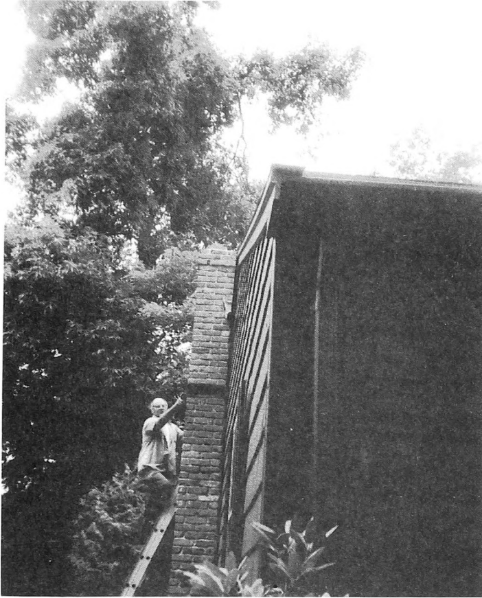
Fig. 4-14. The author checks the condition of a metal strap that is being used to prevent further movement in this chimney.
