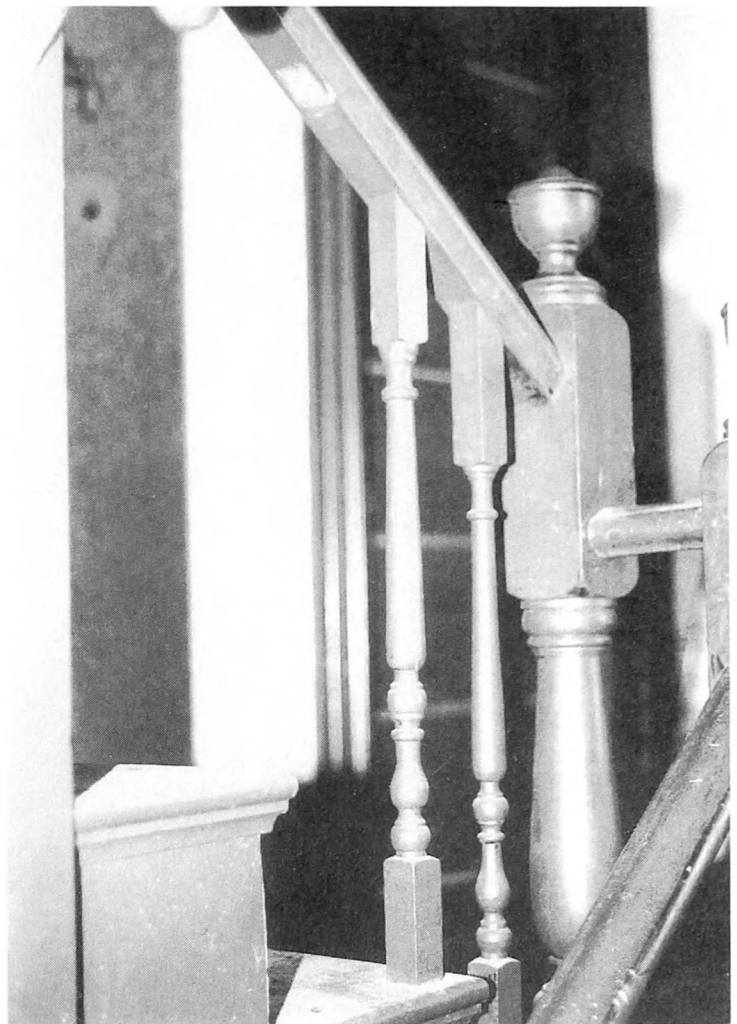
Fig. 8-27. Missing portions of stair rails should be replaced or secured to prevent anyone (particularly a child) from falling through.
