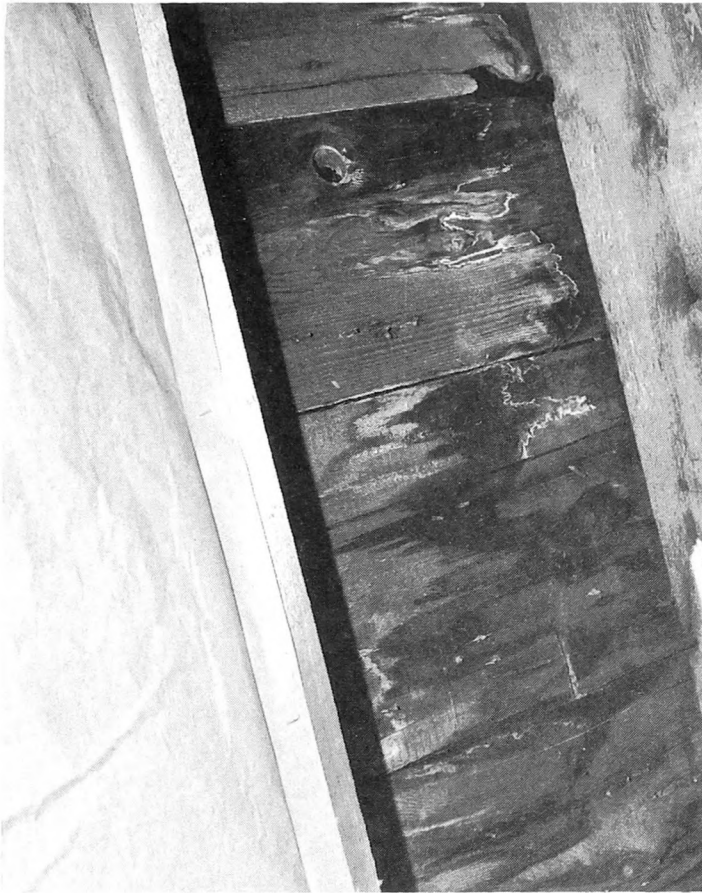
Fig. 4-26. During and after heavy rains, check the attic valley framing areas for signs of water. In this photograph you can see where roofing cement has been applied to keep out water.
