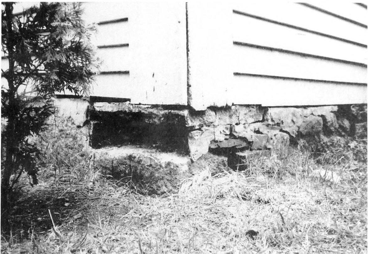
Fig. 2-15. You will need more mortar to fill in the open joints and gaps in deteriorated stone foundation walls, but the principle is the same. Use chinks of small stones to fill in larger openings, then cement them in place.
