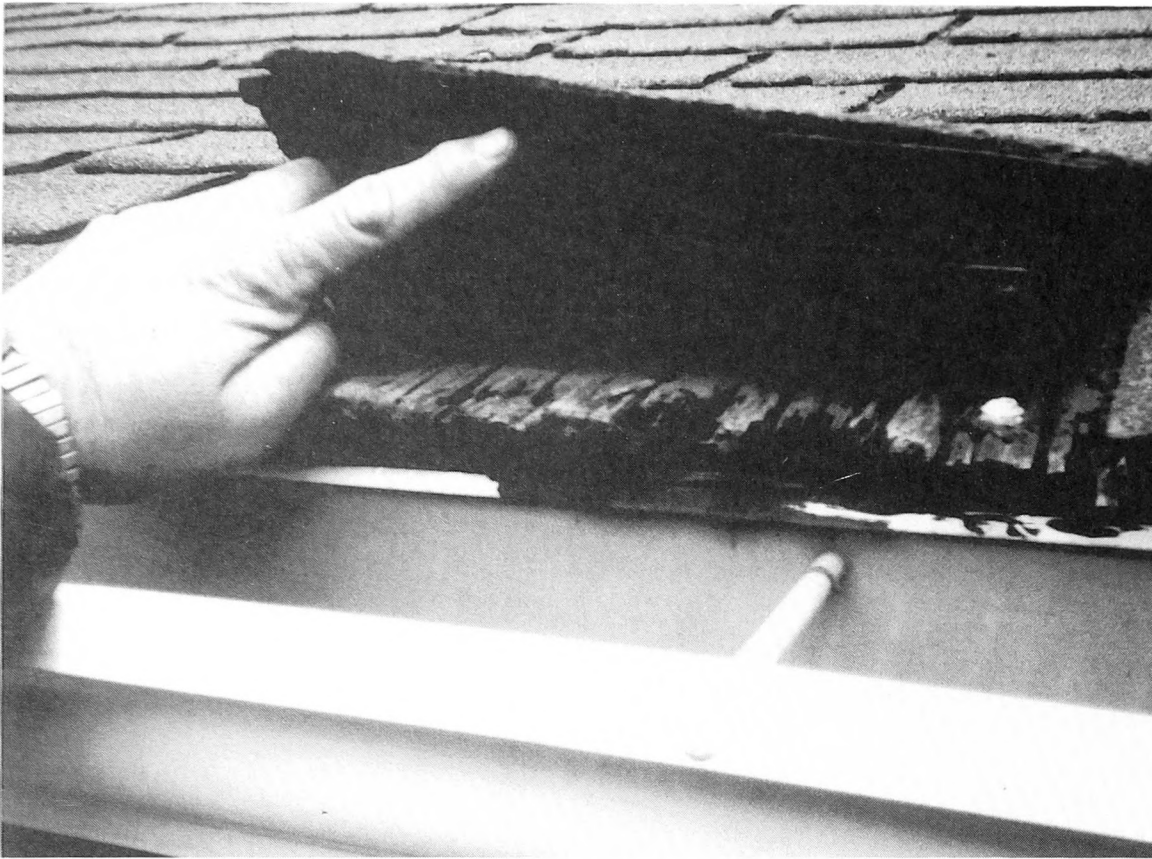
Fig. 5-5. Wood starter shingles at the eaves tend to rot out over the years. When reroofing, insist on replacing this starter edge.
