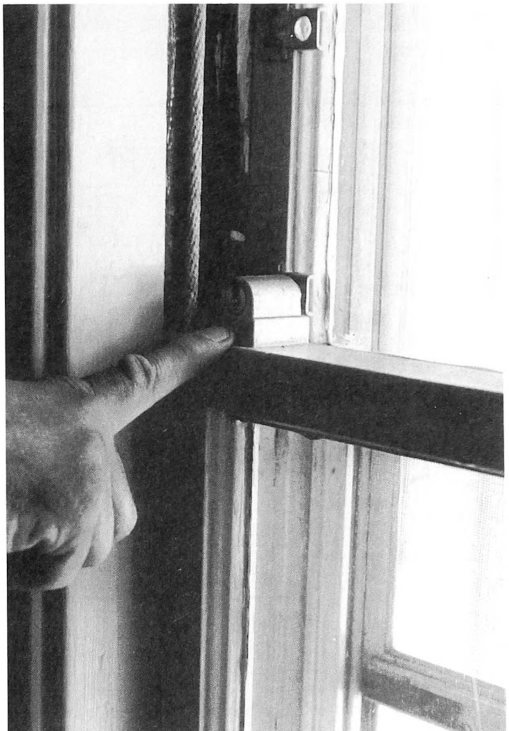
Fig. 8-21. Locks on windows are a stumbling block for burglars, and although they might not deter someone from breaking in, they certainly will slow them up.
