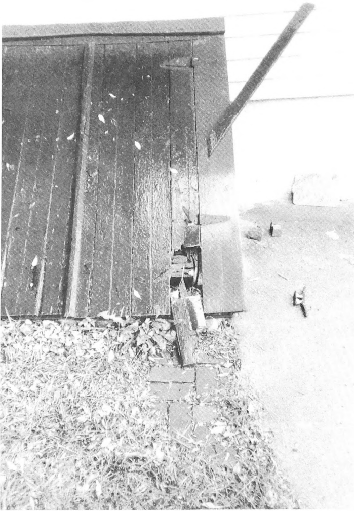
Fig. 1-9. Annual maintenance of bulkheads is crucial in avoiding water in your basements and wood-boring insects in the framing.
