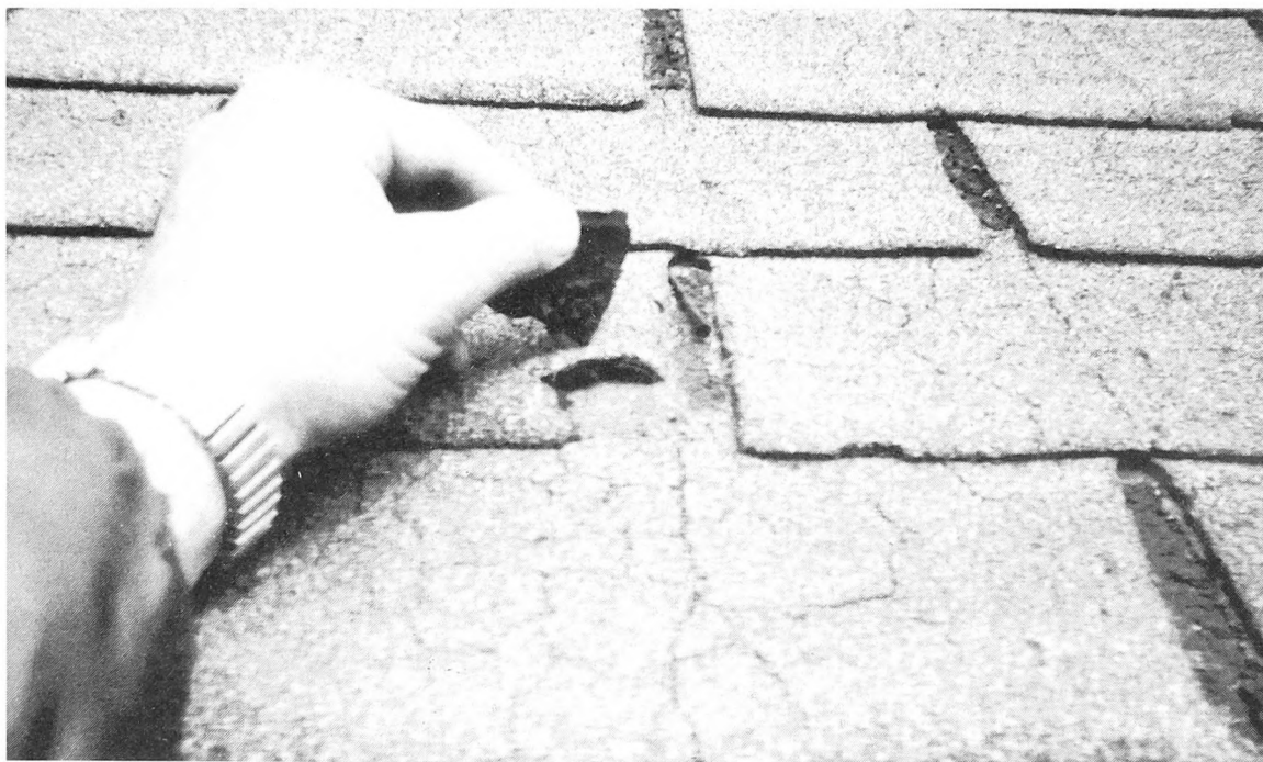
Fig. 1-1. A closeup of roof shingles in advanced stages of deterioration. This roof is ready for replacement.
