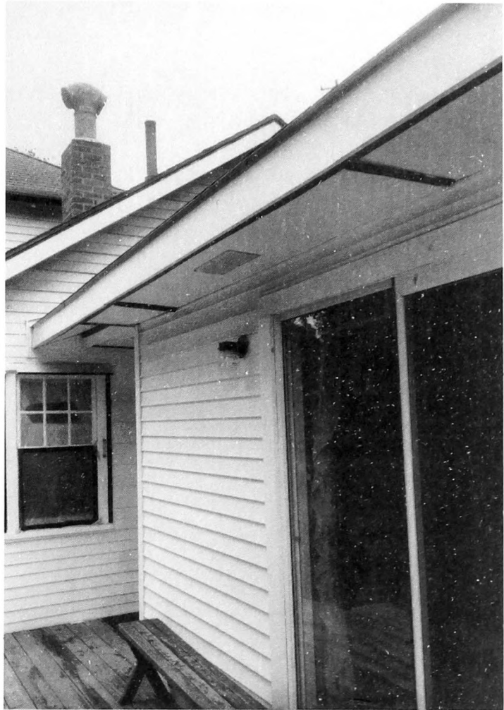
Fig. 2-2. Missing gutters will result in water in basements, erosion of foundation soil, and damage to low wood siding and trim.
